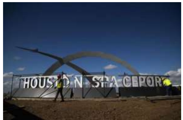
The entrance sign of the Houston Spaceport is being installed by workers.
