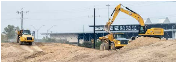
Heavy equipment prepares the future site of Port San Antonio's vertiport in November. Credit: Port San Antonio.
