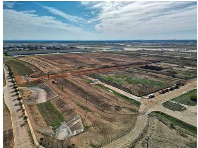
Site work on the Port's new consolidated air services facility began in 2024. Credit: Port San Antonio.
