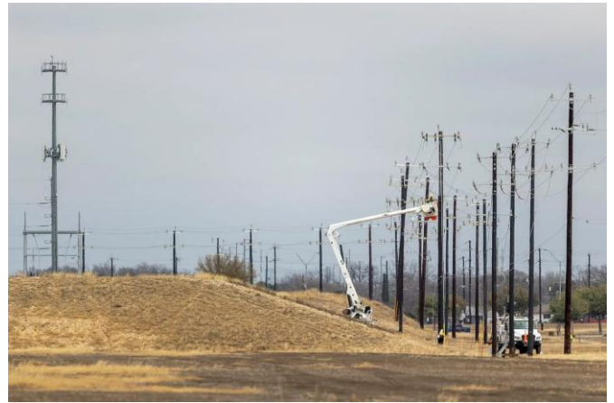
Power lines are being removed and placed underground as the port works to clear out any obstacles for the next generation of aircraft that will be flying in and out of the future vertiport. Image credit: Andrew J. Whitaker/San Antonio Express-News
